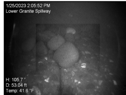
A11 PHOTO: MATERIAL WITHIN CONCRETE JOINT SCALE: 1"=1' FULL SIZE
