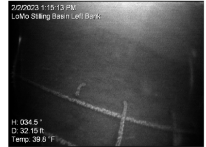
F16 PHOTO: EXPOSED REBAR CAGE AND HOOK
