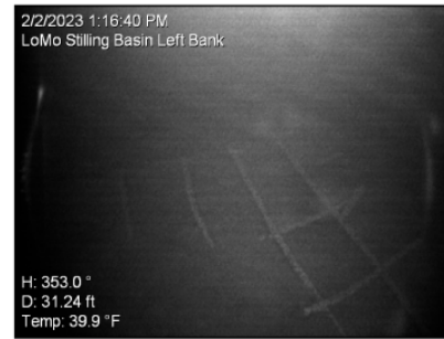
A11 PHOTO: EXPOSED REBAR CAGE
