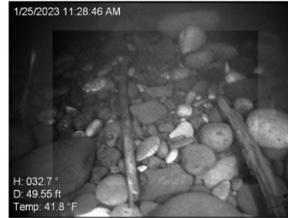
F11 PHOTO: TYPICAL MATERIAL TO REMOVE SCALE: 1"=1' FULL SIZE
